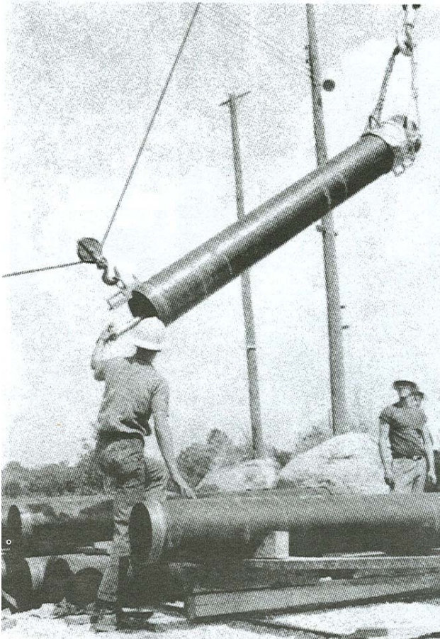
Fig. 7-6. Dragline Guiding Lower End Of Column Section As Column Section Is Being Lifted.
